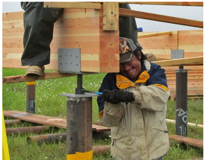
The future homeowners learned the skills needed to operate the homes, such as seasonally leveling the foundation to respond to the dynamic ground.
