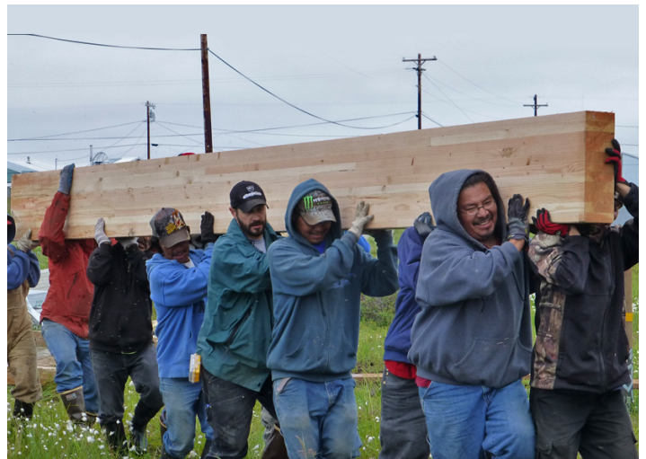
The Atmautluak Traditional Council founded the Pikat Construction Company and hired a local project manager and an all-local construction crew.
