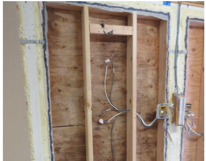
Figure 2. Unsurprisingly, the wall with 2 inches of exterior EPS grew mold after 2 years. This is a common retrofit technique in Fairbanks and occurred in more than 60% of wall retrofits between 1996-2015.
