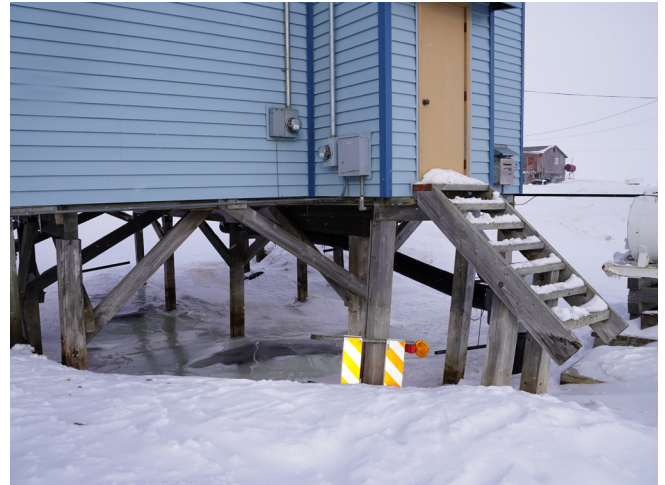
Home shifting due to permafrost
