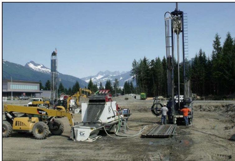
Drilling to establish the vertical ground loops at the Juneau Dimond Park Aquatic Center
